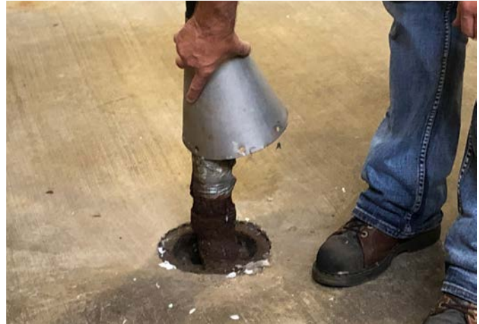
Makeshift sewer gas repair in shower area
