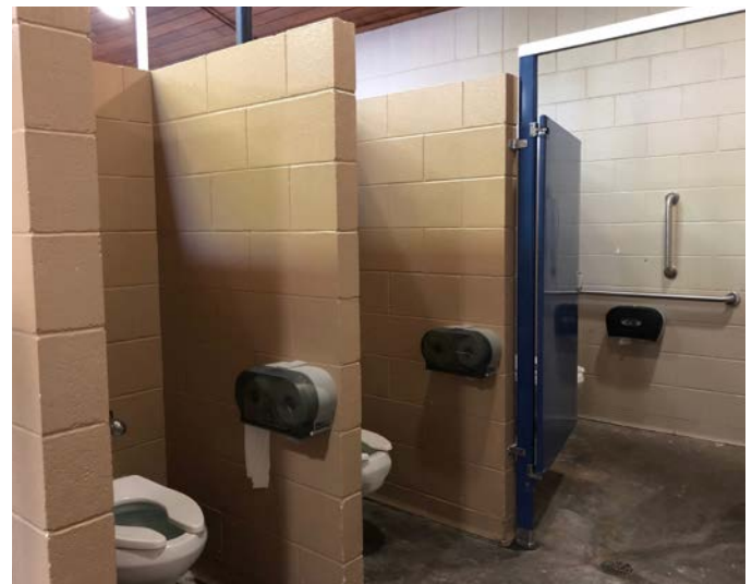
Existing toilet rooms that lacks privacy screening
