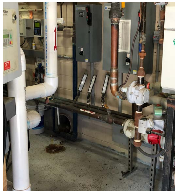
Existing service panels
