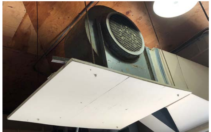
Outdated exhaust fan
